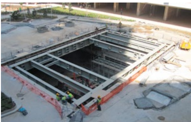
Left: Integrated lighting panels in situ in the open Store.
